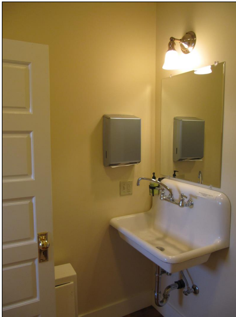
16 of 16 photos WA_Columbia County_Smith Hollow School_0016.tif Bathroom off hallway to office, looking west in 2015
