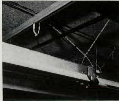
TROLLEY DUCTS run across on 16 ft. centers. Each fixture plugs in separately.
