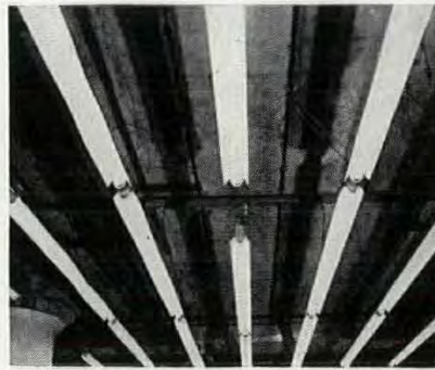
FLUORESCENT LAMPS hang from channels embedded in concrete floor slab.
