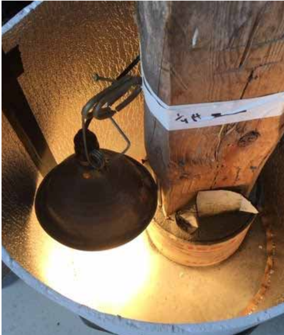
As winter came on, support piers were poured, insulated and heated long enough for the concrete to cure.
