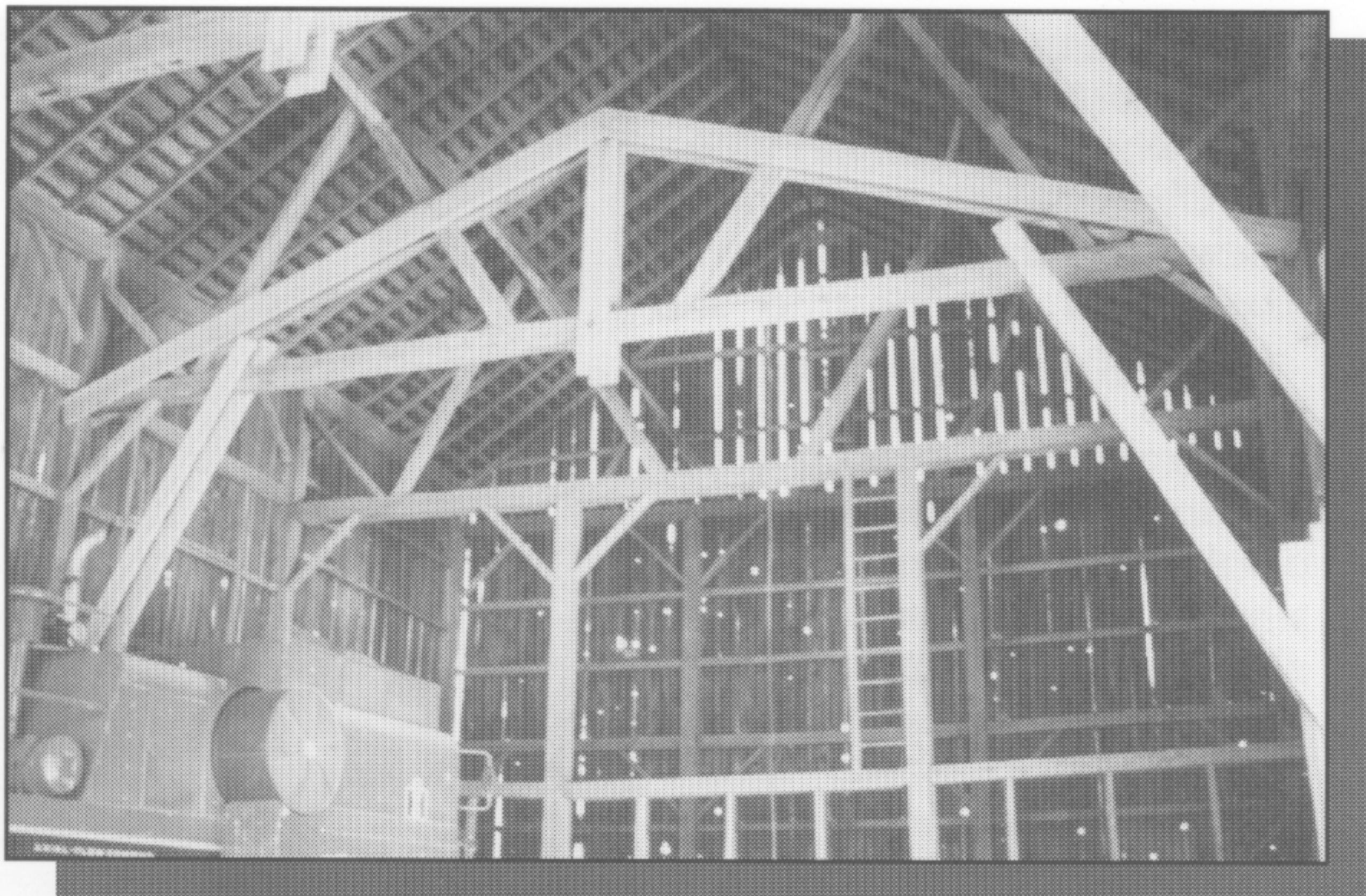
Interior of Newton barn, showing new truss and knee braces (foreground) and original post and beam structure (background)
