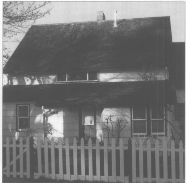
Historically, wood shingles were used on most structures. Many have been replaced with composition shingles.
