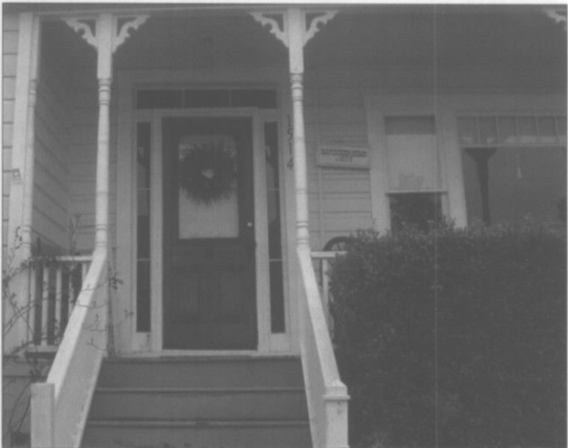
Protect and maintain significant stylistic features, such as these windows, eave trim and porch columns and railings. (Steilacoom, WA)
