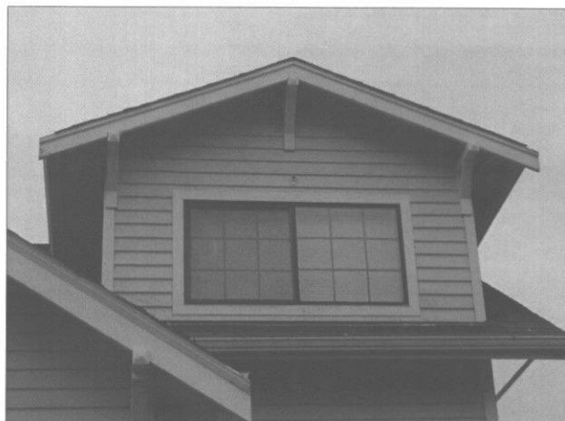
Preserve the original eave depth. The shadows created by traditional overhangs contribute to one's perception of the building's historic scale. (Steilacoom, WA)
