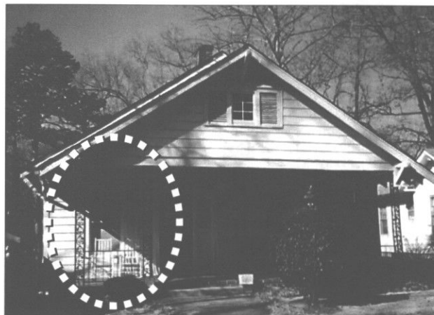
Inappropriate: This porch has experienced an inappropriate alteration; wrought iron supports have replaced wood piers. Compare it with its “twin” in the photo below. (Spartanburg, SC)
