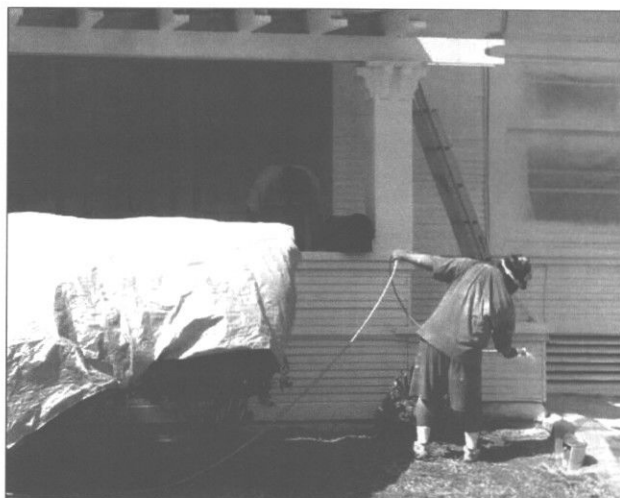
Protect wood siding and other wood surfaces with a painted finish. (San Jose, CA)
