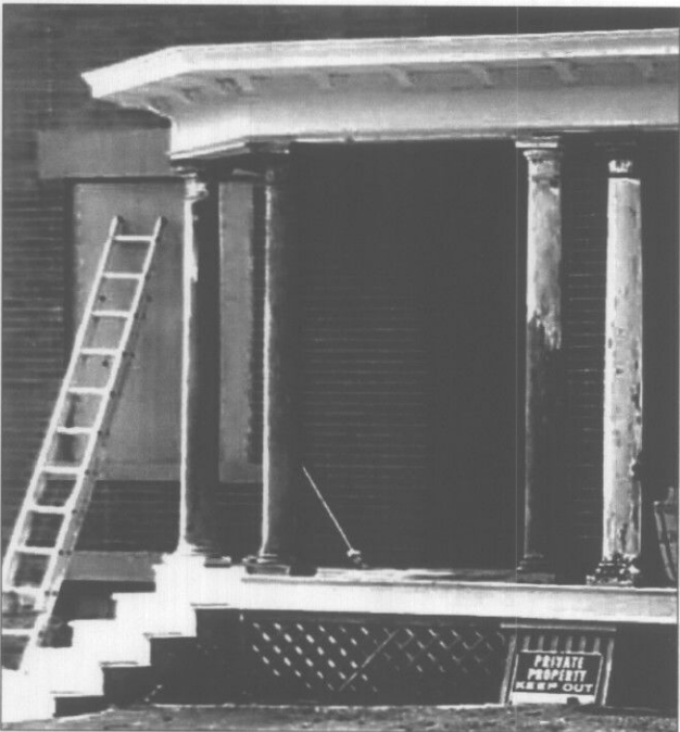
Repairing rather than replacing porch elements always is the preferred approach. (Washington, MO)
