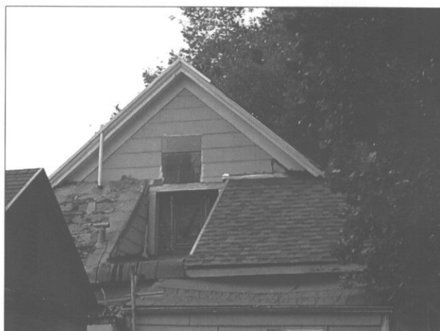
Look for breaks or holes in the roof surface, and check the flashing for open seams. (Sacramento, CA)
