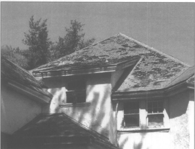
Roof materials are the most susceptible to deterioration, and their replacement may become necessary in time. (San Jose, CA)
