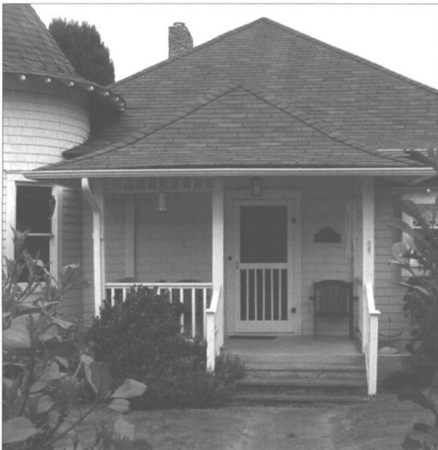
Windows and doors are some of the most important character-defining features of a structure. (Steilacoom, WA)
