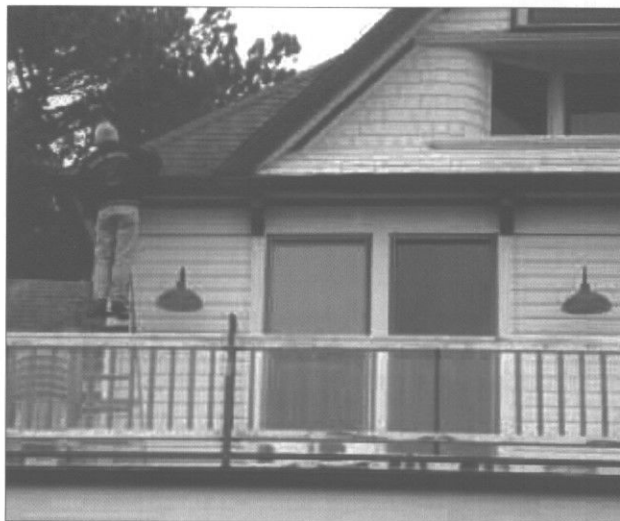
Regular maintenance and cleaning is the best way to keep a roof in good shape. (Steilacoom, WA)
