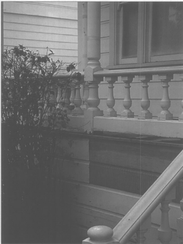
Appropriate: Repair wood features by patching or piecing-in new wood elements that match the original. (Sacramento, CA)
