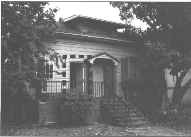
Inappropriate: Do not add new window or door openings on character-defining facades. (San Jose, CA)
