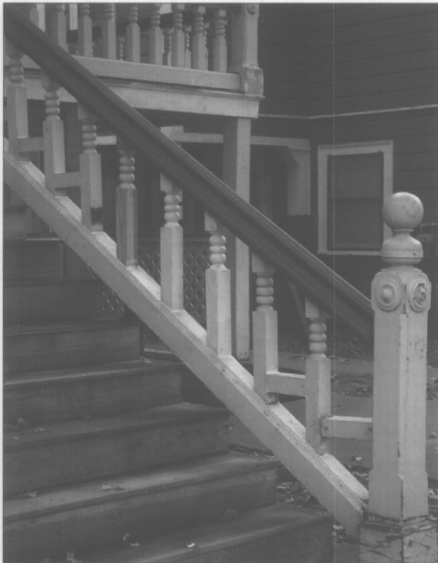
Repair deteriorated, primary building materials by patching, piecing-in, consolidating or otherwise reinforcing them. (Sacramento, CA)
