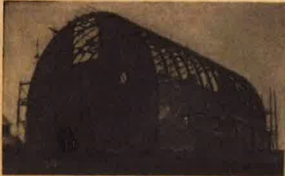
Circle roof barn of Mr. N. V. Anderson, Cowles, Nebraska, under construction.
