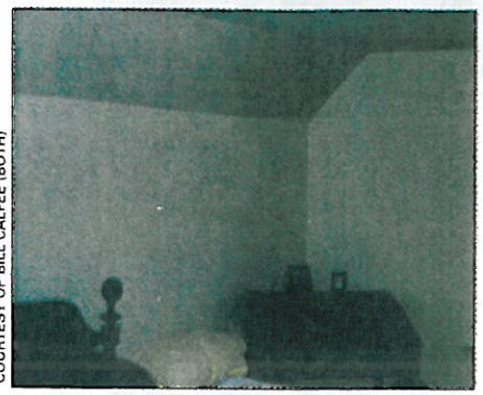
An audit photo shows cold spots where insulation is lacking in an exterior wall—a good place to add fiberglass batts if opportunities for access ever present themselves.
