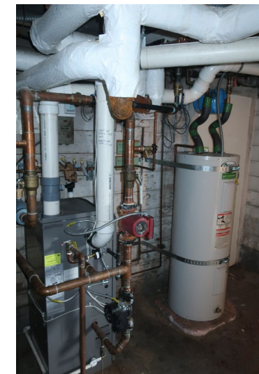
Figure 171. View looking southeast at the boiler and hot water heater.
