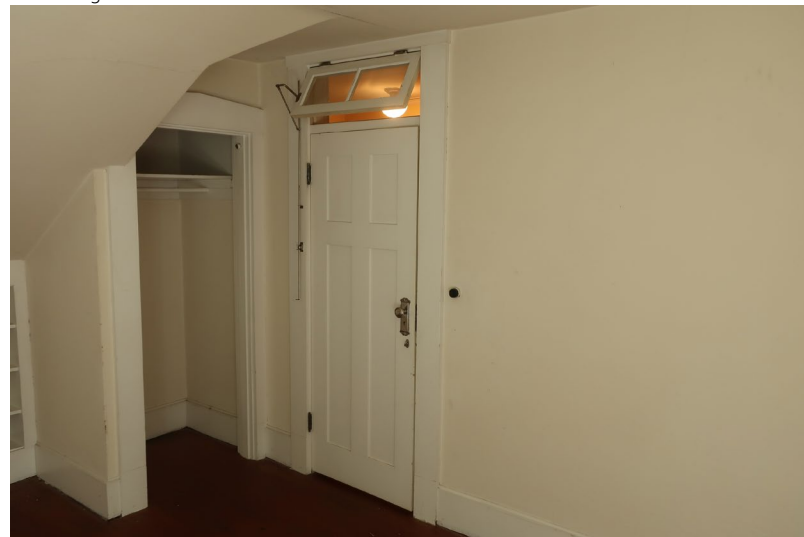
Figure 322. View looking northwest at closet and hall door, with multiple roof /ceiling angles.
