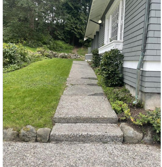
Figure 66. Concrete steps and walkway along the east side, looking south from the driveway. Repairs can be seen particularly along the west (right) edge.
