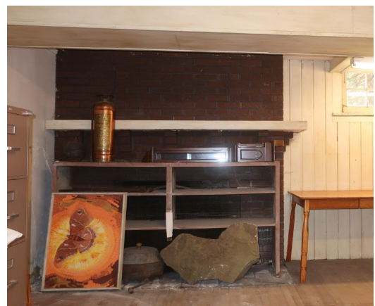
Figure 90. Detail of disused fireplace in the Northeast Room, with brick surround to the ceiling, and raised stone hearth on the raised wood floor. There is water damage on the adjacent wall to the left.
