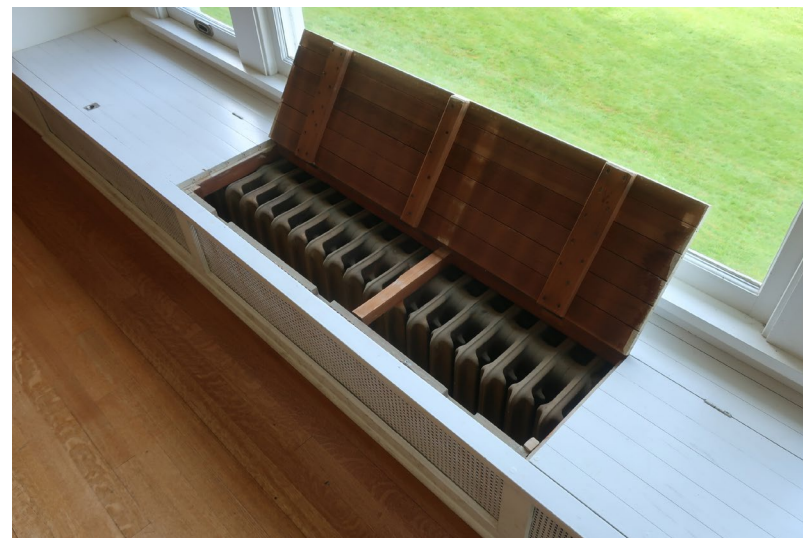
Figure 287. Detail of the radiator bench and access in the west bay window.
