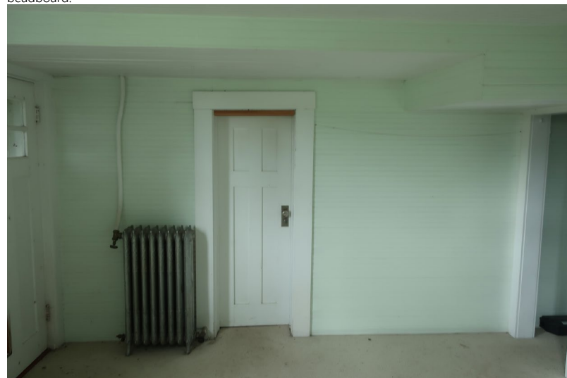
Figure 133. View looking north at the Bathroom door, and two levels of soffits. Ceiling heights are very low, especially with the raised floor..
