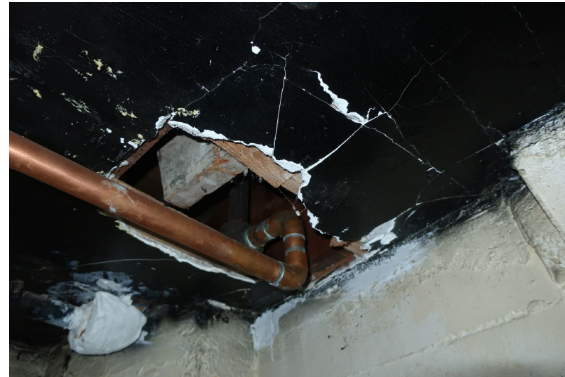
Figure 202. Detail of copper piping extending through plaster ceiling to radiator above.
