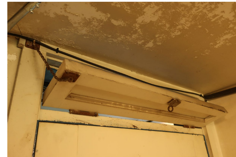
Figure 187. Detail of operable solid-panel transom over the door. Note the paint condition on the plaster, which is typical heavy flaking, due to the high humidity of the space.
