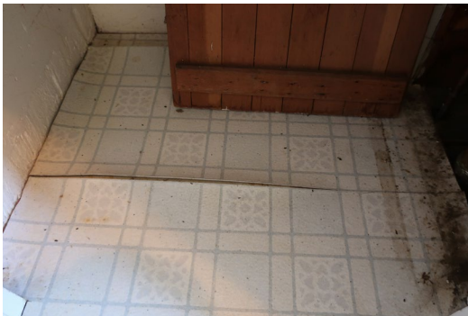
Figure 79. Sheet linoleum flooring at the Second Floor Bath 3, peeling up and heavily soiled. It is likely that most of the sheet flooring products at the restrooms are not original.
