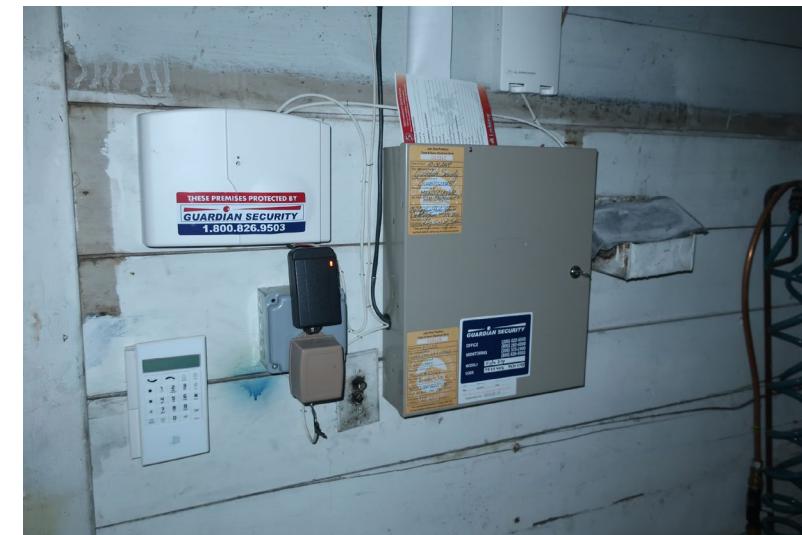
Figure 169. Detail of security system on north wall.
