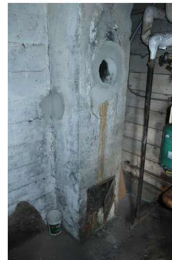
Figure 172. Detail of the chimney with cleanout and breach..
