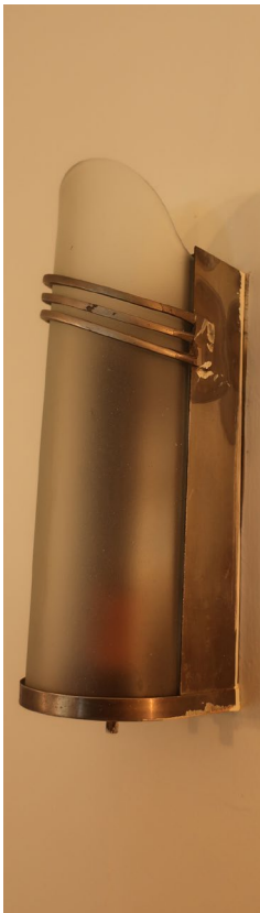
Figure 102. Original light fixture detail.
