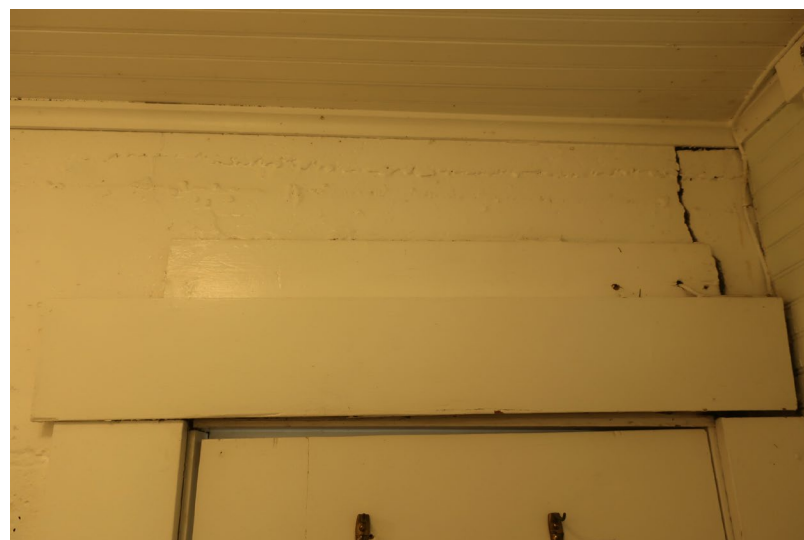
Figure 144. Detail concrete crack above door head.
