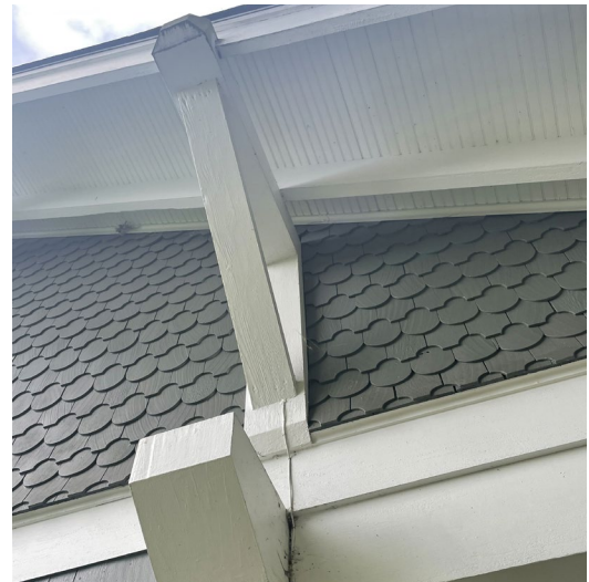
Figure 59. Detail of south facade half-cove shingled gable, knee brackets, and exposed rafters.
