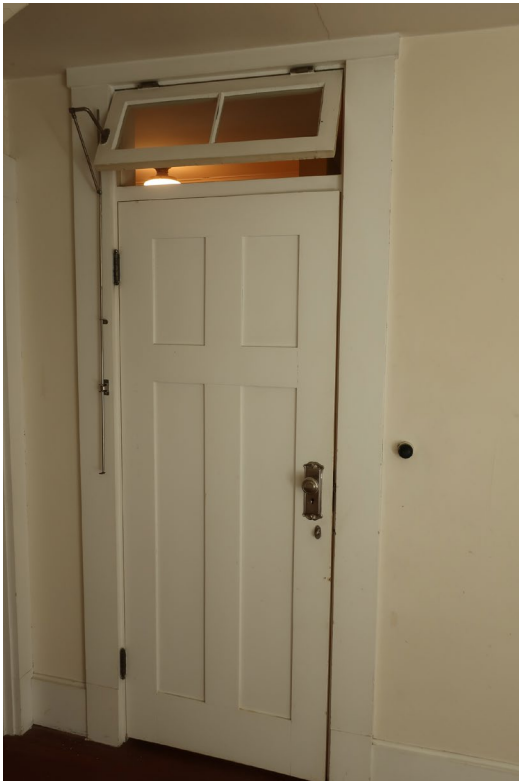
Figure 86. Typical painted wood 4-panel door. This one is at Second Floor Room 1 (in the original part of the house), and has an operable glazed transom.
