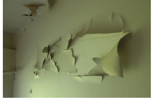
Figure 82. Paint peeling at plaster wall and ceiling in Bath 4. This is a fairly extreme example, not typical, but more prevalent in the humid restrooms where the hard enamel paint has debonded in sheets.
