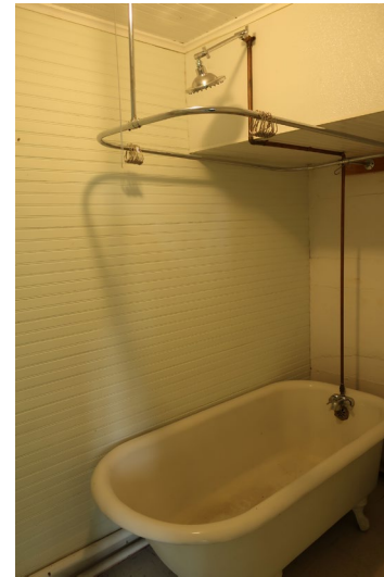
Figure 141. View looking northeast at clawfoot tub, FRP-wrapped soffit, and exposed piping.
