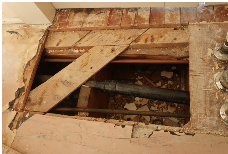
Figure 332. Access hole into the floor cavity.
