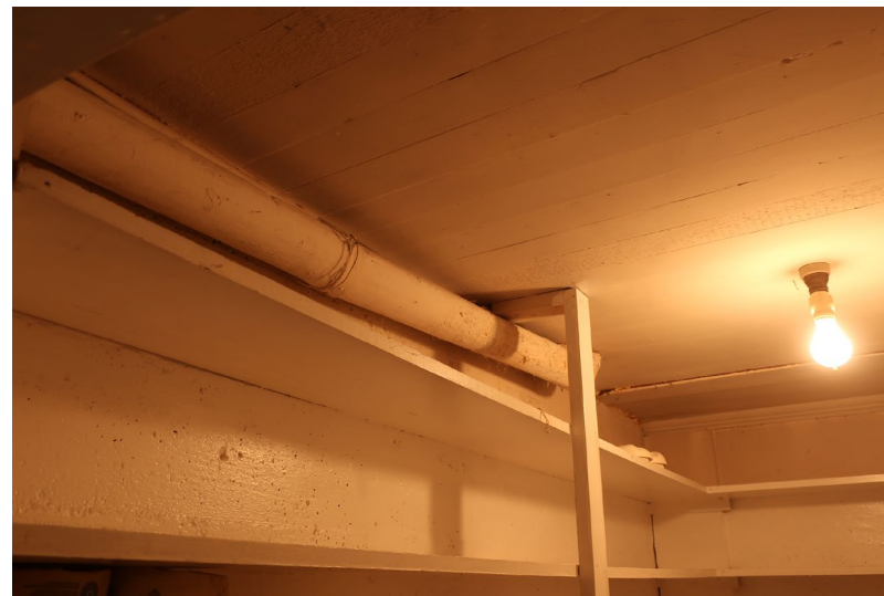
Figure 125. Detail of T&G ceiling, insulated radiator piping, and bare bulb light fixture.
