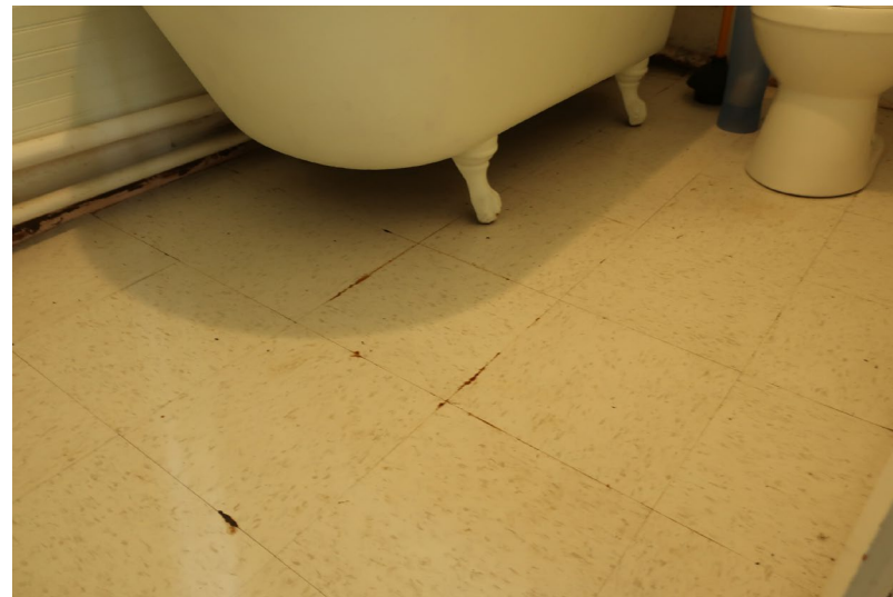
Figure 143. Detail of VCT flooring, clawfoot tub, and surface mounted piping on the wall base.
