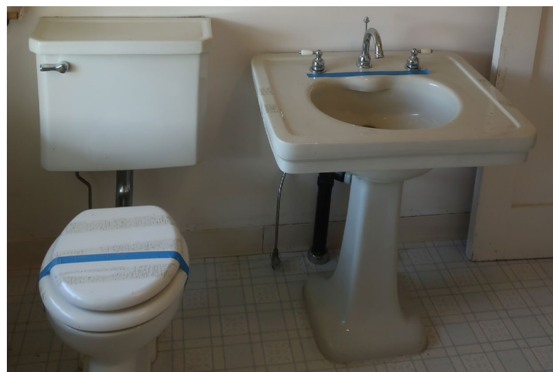
Figure 366. Detail of decommissioned sink and toilet.
