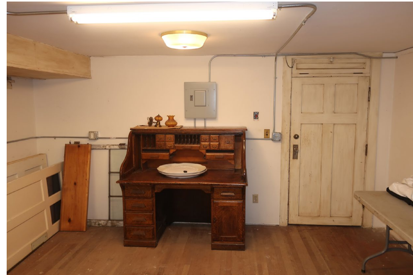
Figure 193. View looking south. Lighting and power has been surface mounted to walls and ceilings.
