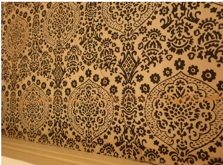
Figure 81. Wall paper in the Original Dining Room, with horizontal wear marks at the plate rail, and telegraphing cracks at the underlying plaster substrate.
