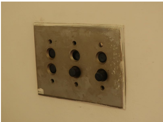
Figure 63. Detail of push button light switch.
