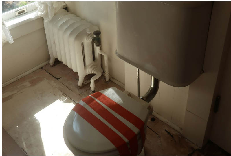
Figure 330. Plumbing fixtures have been decommissioned to control waste water load.
