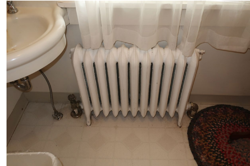
Figure 243. Detail of cast iron radiator and linoleum sheet flooring, with rubber wall base.
