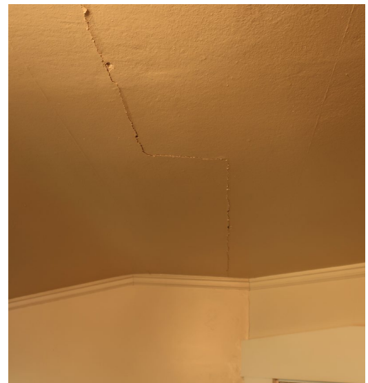
Figure 84. Plaster ceiling crack at Second Floor Room 2, likely telegraphing movement in the structure at some time.
