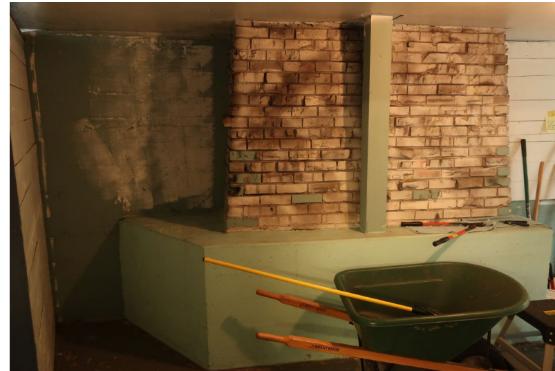
Figure 158. Detail of original exterior brick chimney with tall concrete plinth. New framing supports the addition floor.
