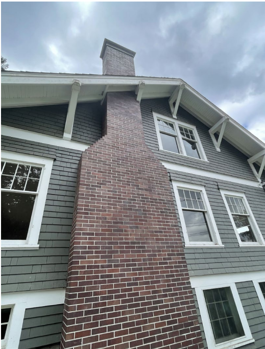
Figure 70. Detail of the north chimney. Prior crack repair was observed at the lower east corner, near the cleanout.
