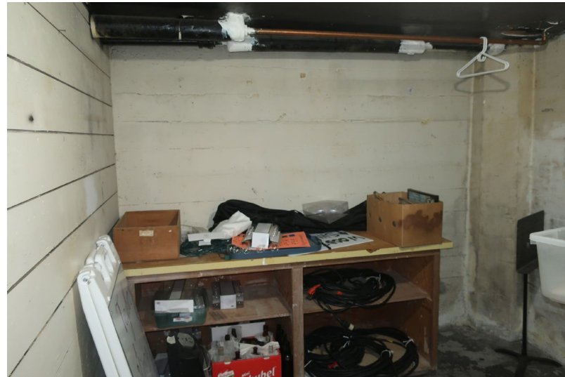
Figure 201. View looking east at the concrete foundation / retaining wall. Partially insulated copper radiator piping is visible at the ceiling.
