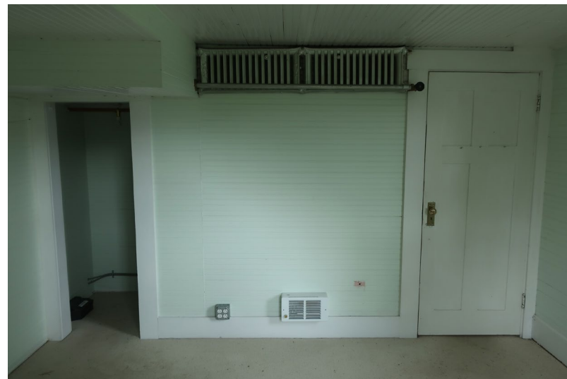
Figure 134. View looking east. The opening to the closet is at left, and door to the Kitchen is on the right. Note the wall mounted cast iron radiator, and low wall unit heater.
