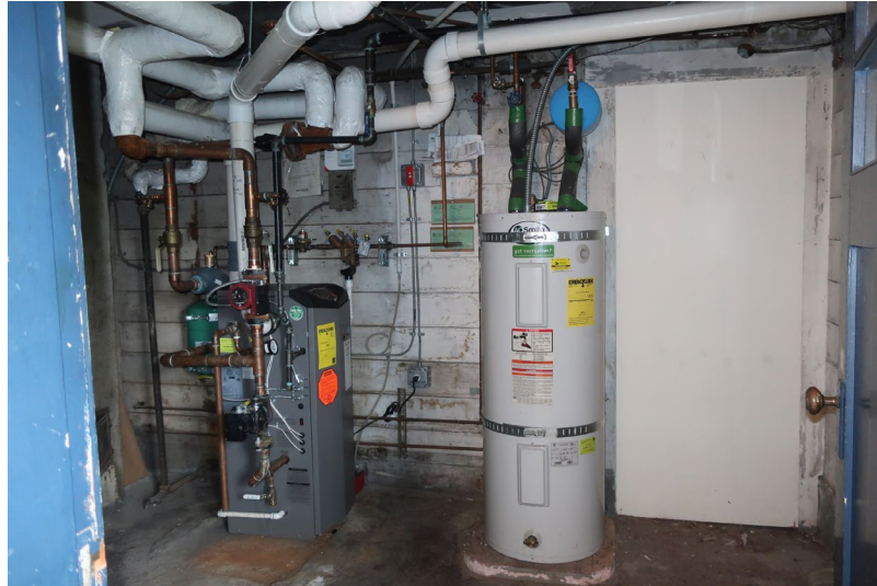
Figure 165. View looking south. Original exterior door at right has been closed up.
