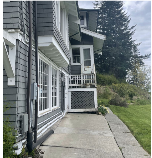
Figure 67. Concrete walkway along the west side, looking south. Exposed electrical conduit, disconnects, and other appurtenances are surface-mounted along the west wall, and extend up the northwest corner, creating visual clutter on a prominent corner.
