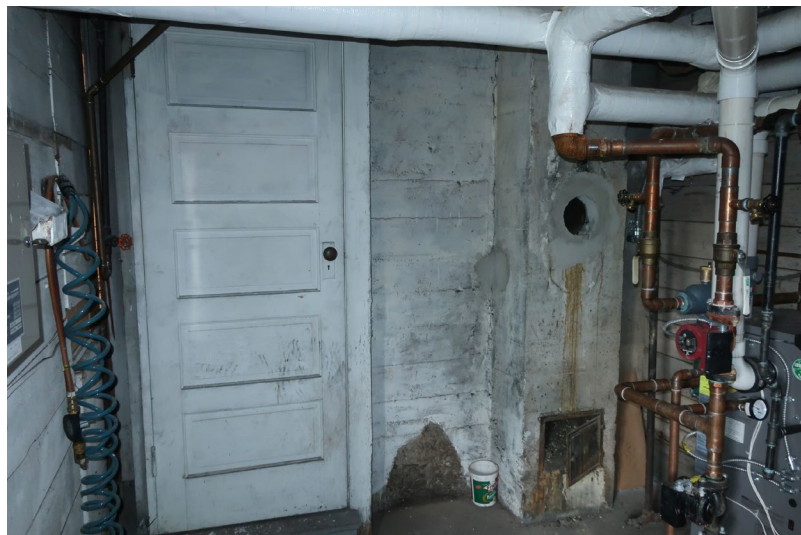
Figure 168. View looking east, at door to the Basement stair at left, and the concrete chimney base that served the original boiler and the Kitchen stove above. Note the concrete spall at the wall base.
