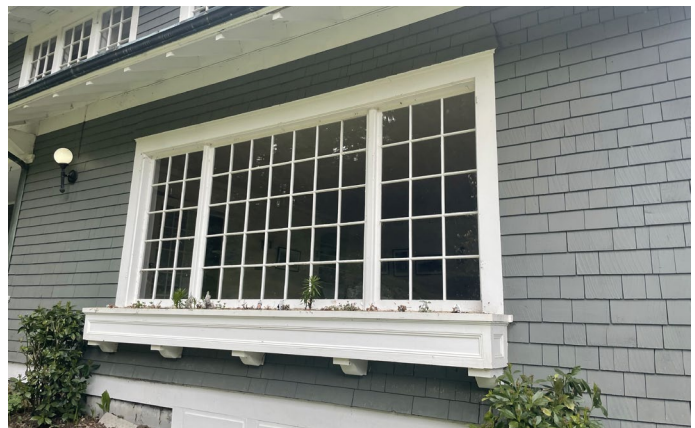
Figure 71. Detail of large east window in the Living Room. This window replaced the original 4-ganged double-hung assembly, and has been recently repaired after damage from an impact broke several panes and muntins. The flower box with brackets and exterior light fixture appear to be original.
