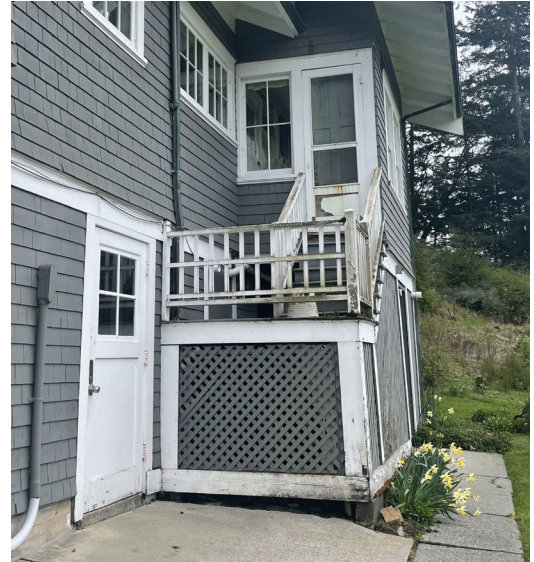
Figure 74. Detail of the west exterior stair, looking south. Paint failure and rotted wood on the decking and railings are evident.
