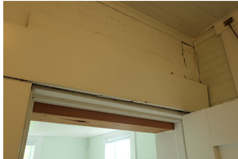
Figure 140. Detail of door head with framing repair, and concrete crack visible at upper right corner.
