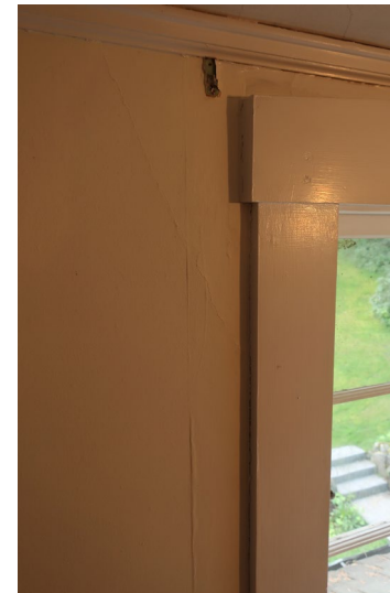
Figure 405. Detail plaster crack
