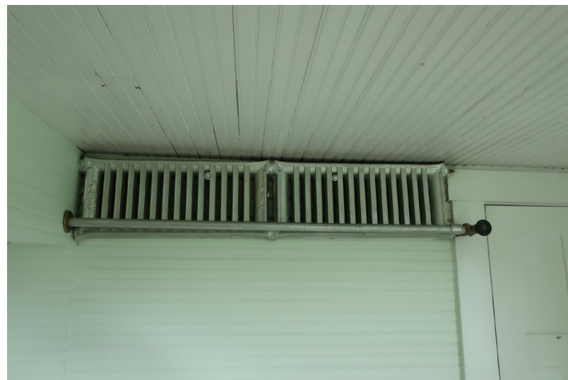
Figure 135. Detail of wall mounted cast iron radiator.
