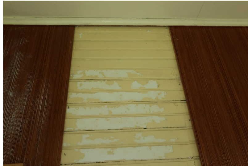
Figure 269. Detail of the rilled panelling, and what appears to be a missing panel over painted beadboard siding.
