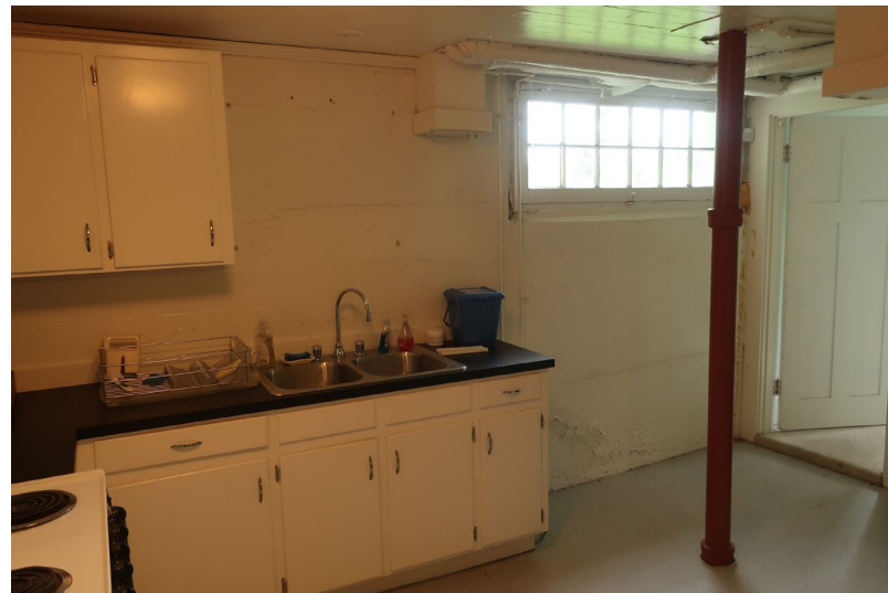
Figure 116. View looking south with a waste pipe stack (red) in the middle of the space, and a high-silled window. The Bedroom door is at right..
