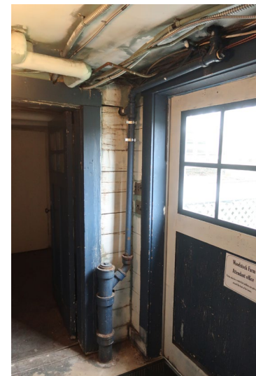
Figure 163. View of exterior door at west, with waste stack, and extensive wiring at the ceiling..
