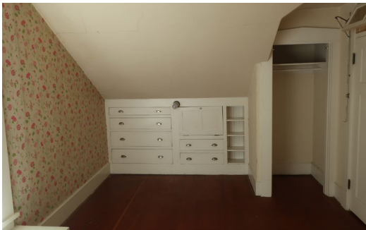
Figure 50. Room 1 looking west with sloped plaster ceiling and built-in wardrobe in the knee wall. This original bedroom also has an operable glass transom to the hall.
