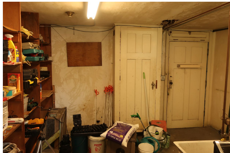
Figure 186. View looking south. A built-in cabinet is at center, and the entry door with transom is at right. An original light fixture is visible adjacent to a contemporary fluorescent strip fixture.
