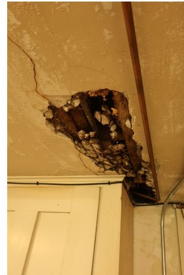
Figure 185. Detail of plaster damage, and possibly prior repair at a plumbing penetration, south end of ceiling.
