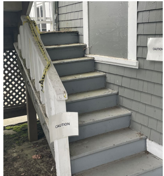
Figure 75. Detail of the west exterior stair, looking northeast. It is currently signed for no access.
