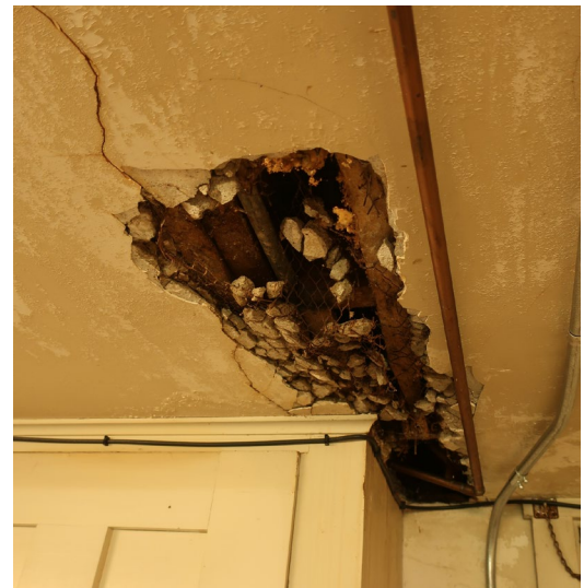
Figure 83. Plaster ceiling damage at the Basement Laundry Room, south wall, either due to water damage, movement, or intentional removal to install or access concealed utilities. Note the opening has both metal and wood lath.
