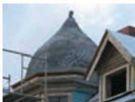
Hays-Hood Turret with water barrier
