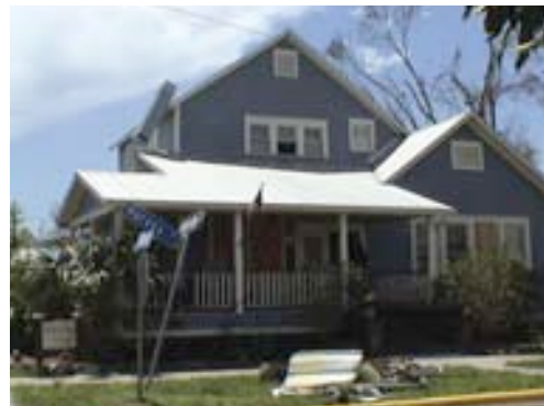
Chimneys are vulnerable roof features that require securing.
