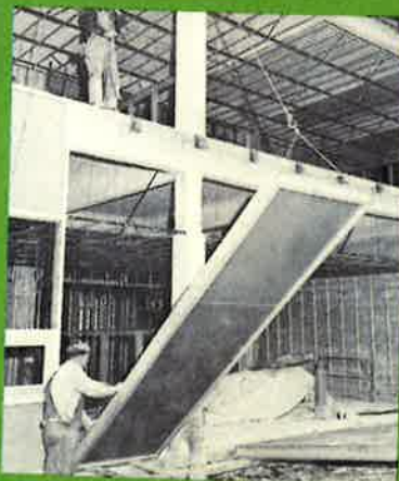
ALASKA MENTAL HOSPITAL under construction. An insulated panel unit being guided into place by Fentron's skilled field men.
