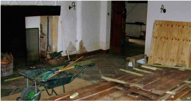
Floorboards carefully stacked at Wickhamford Manor during post flooding repair work. [photo © Peter Rhodes/Ward and Dale Smith]
