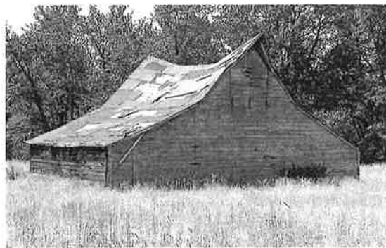
Figure 15. Goodman barn, southern edge of the Gallatin Valley, Montana, construction date unknown. Undersized ridge beam and inadequate cross-bracing have led to structural failure. Photograph by Maire O'Neill Conrad, 2016.
