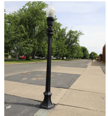
Figure 28. Light Standard B Example. View showing a typical type B light standard
