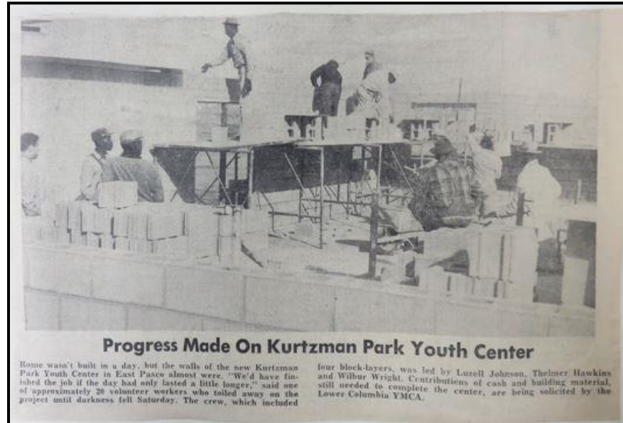
Figure 23. Erecting the walls of Kurtzman Park Youth Center, Tri City Herald , March 2, 1963.
