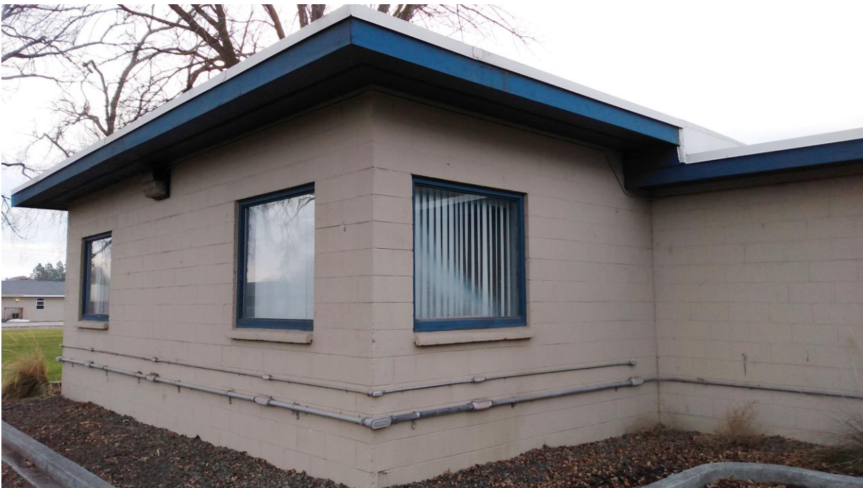
WA_FranklinCo_KurtzmanPark_0005. Looking west to the east (side) wall of the youth center.
