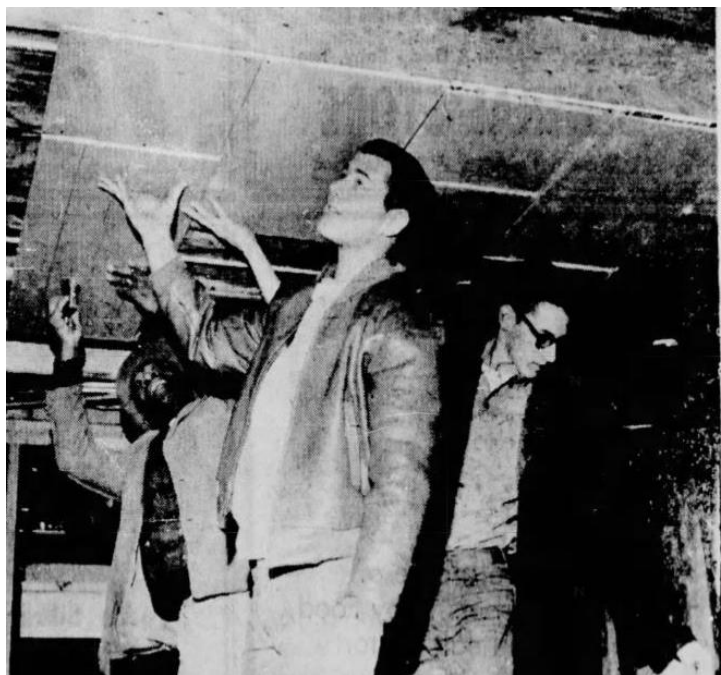
Volunteer workers scramble to finish the inside of Kurtzman Park Youth Center, Tri-City Herald , December 31, 1963.
