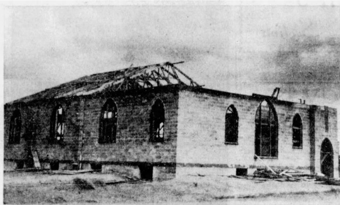
GOING UP — Pasco's new Morning Star Baptist Church building is shown nearing completion at 632 Douglas St. The religious edifice, comprising a full basement and 3,200 square feet of floor space, is expected to be completed in September.
