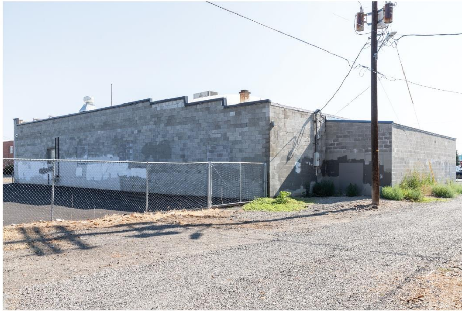
WA_Yakima County_Yakima Valley Filipino Community Hall_0005. Southwest corner viewed from the alley.
