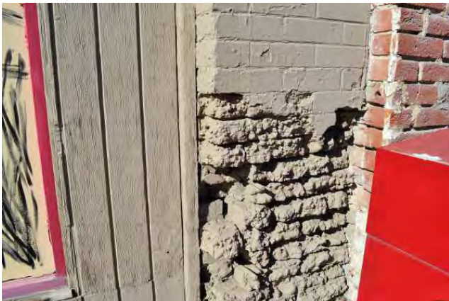
Damaged brick in east pilaster, 2021. View to NE.
