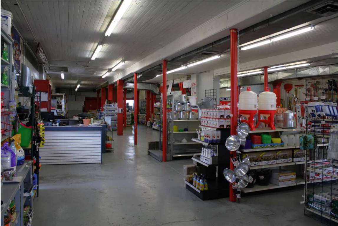
18 of 23. Front half of the interior of the Kennewick Fruit & Produce Co. Building, showing some replacement metal structural posts. Camera facing southwest.
