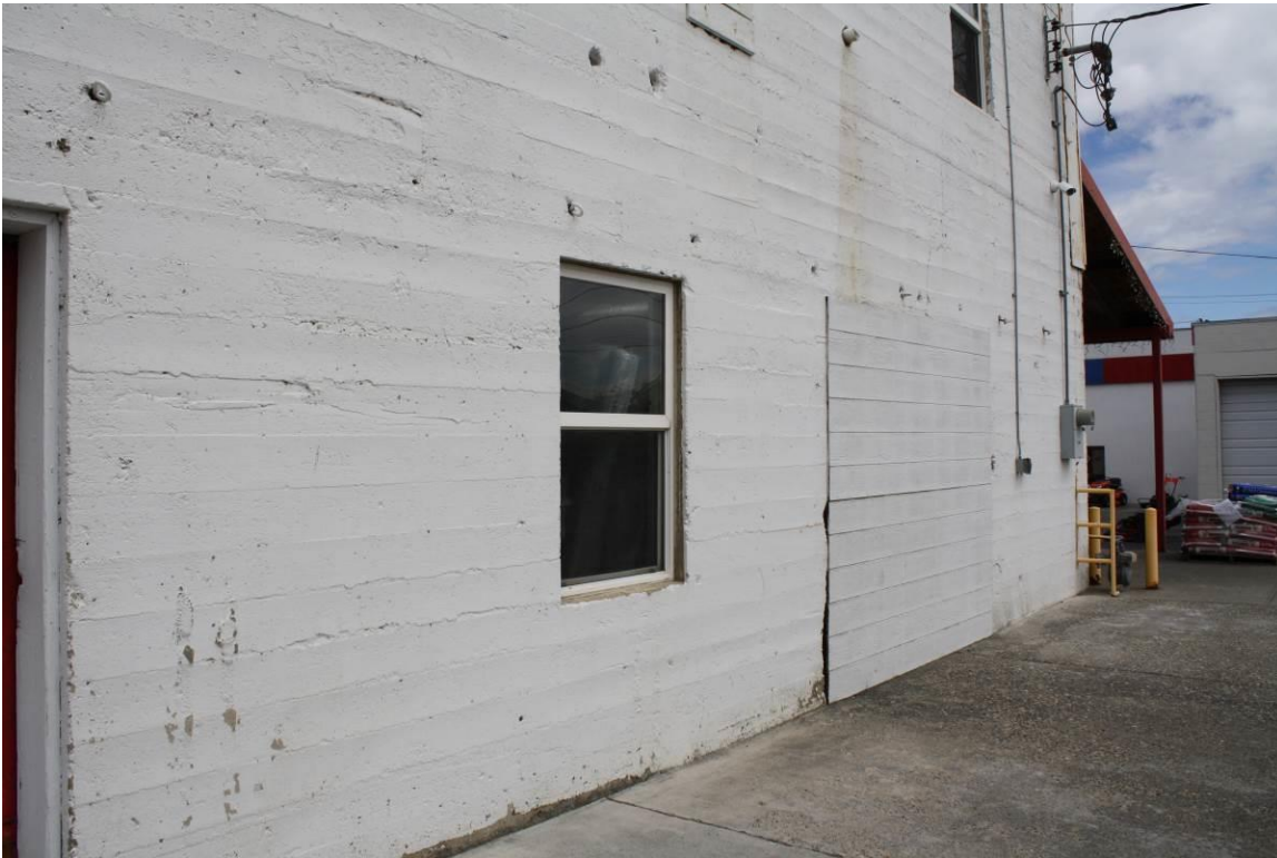
10 of 23. Detail view of replacement fenestration and door opening enclosed with wood boards on south side of the Kennewick Fruit & Produce Co. Building. Camera facing northwest.
