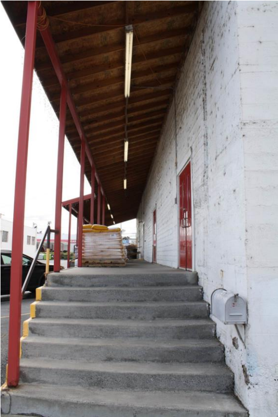
4 of 23. Covered concrete walkway/platform on east side of the Kennewick Fruit & Produce Co. Building. Camera facing south.
