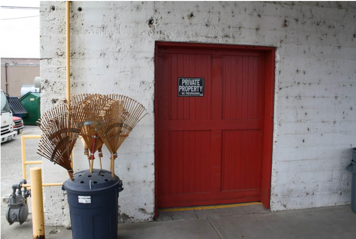
6 of 23. Original wood door on the east side of the Kennewick Fruit & Produce Building near the southeast corner. Camera facing west.
