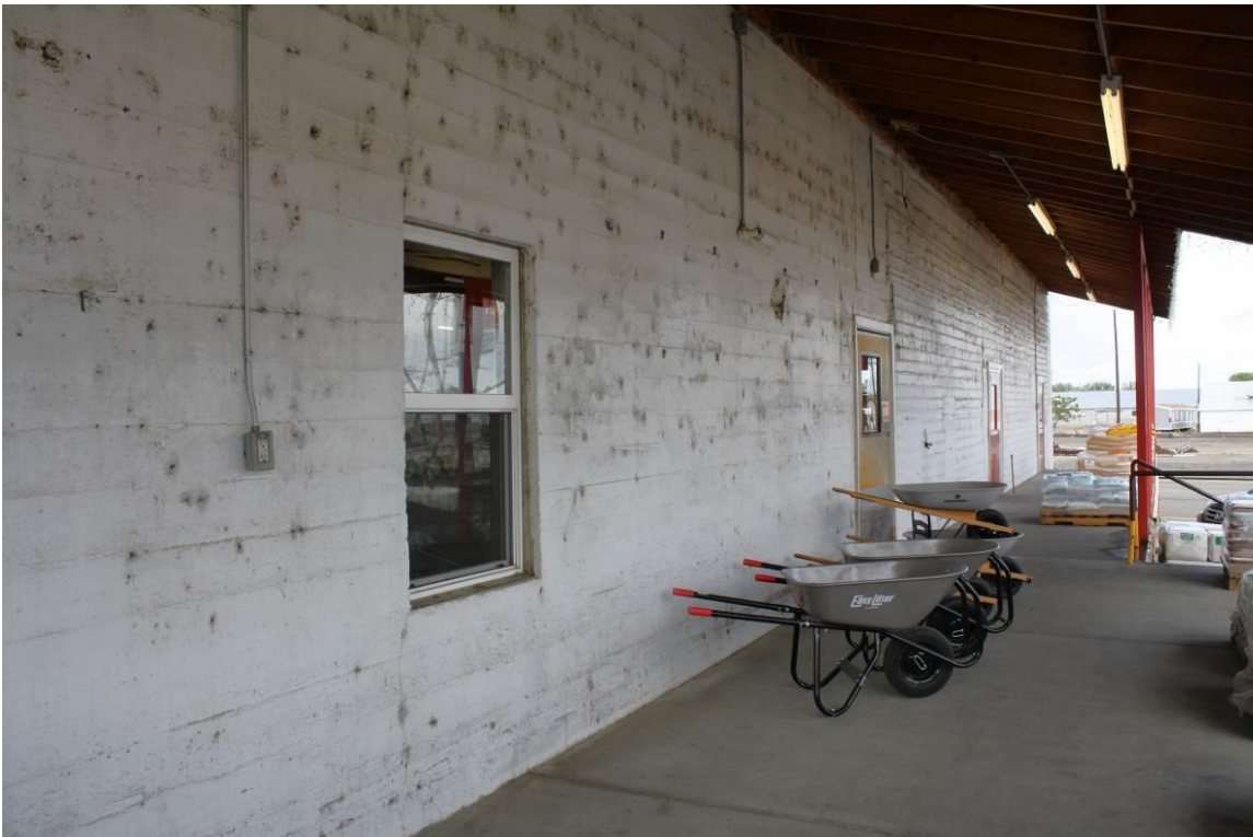
5 of 23. Detail view of replacement fenestration on the east side of the Kennewick Fruit & Produce Co. Building. Camera facing northwest.
