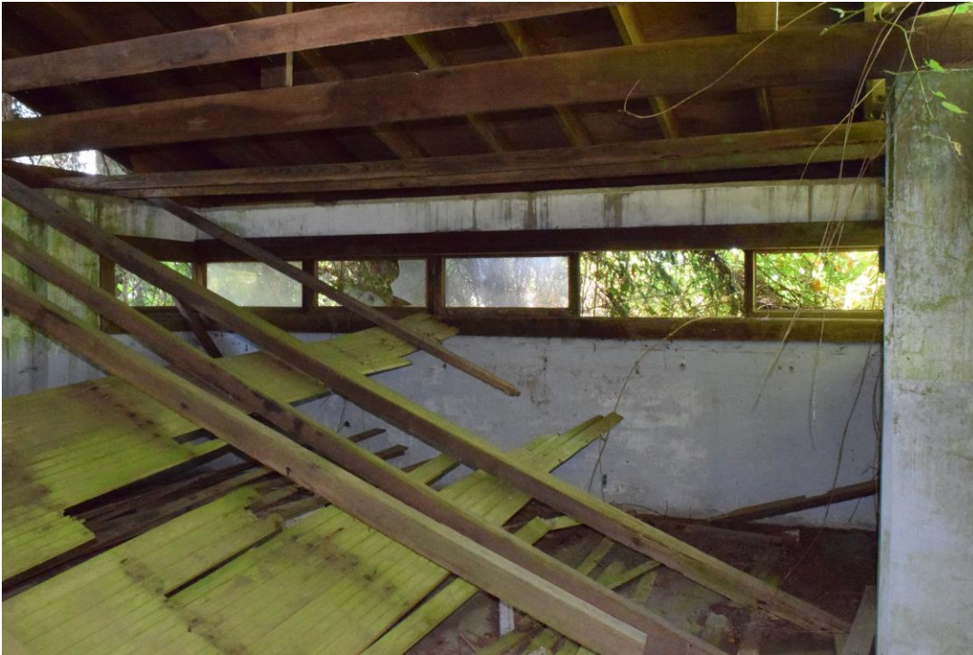
Photo 22. Interior of the Mine Command Station showing collapsed ceiling and observation opening.
