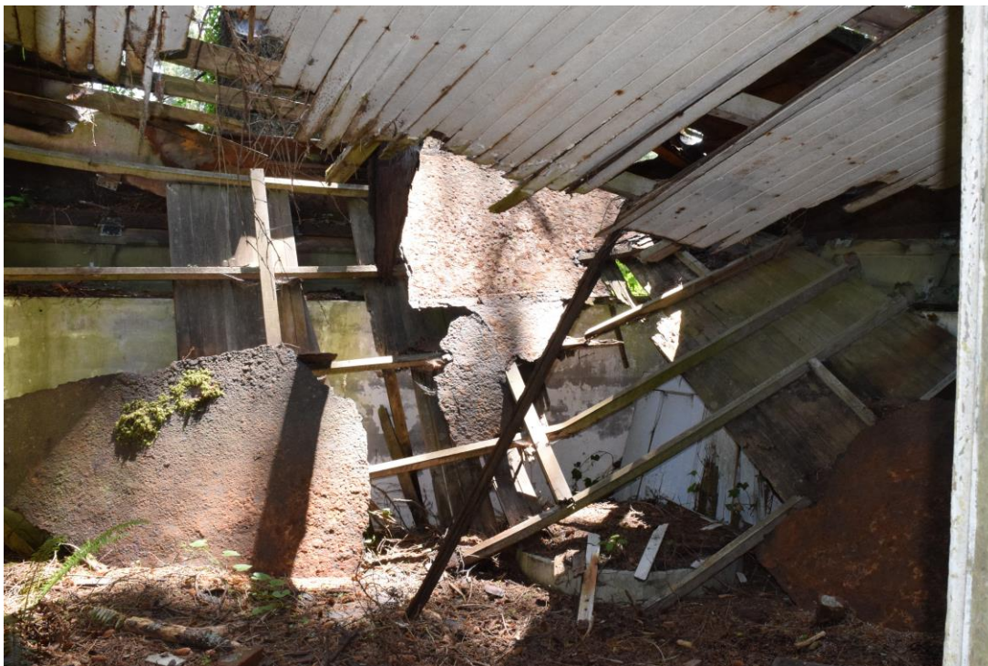
Photo 20. Interior of Site ID No. 29 showing portions of collapsed metal roof and wood ceiling.
