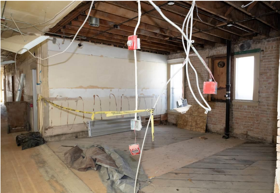
WA_Spokane County_Hotel Collins_0042. Third floor, looking southwest through the former shared bathroom space.
