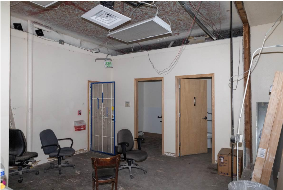
WA_Spokane County_Hotel Collins_0021. First floor, looking southeast towards the alley entrance (left doorway) and the two bathrooms (right doorways).
