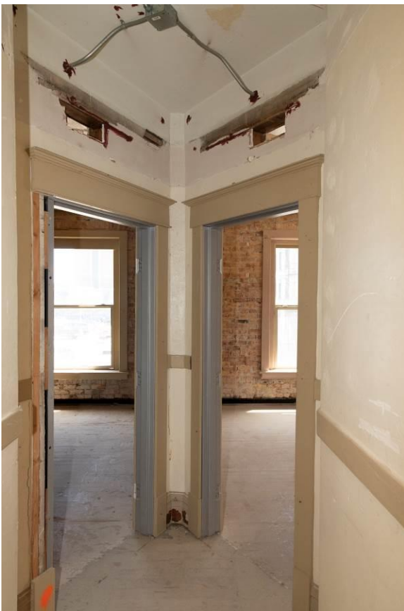
WA_Spokane County_Hotel Collins_0031. Second floor, typical branch hallway showing the angled vestibule at the unit doorways, looking east.
