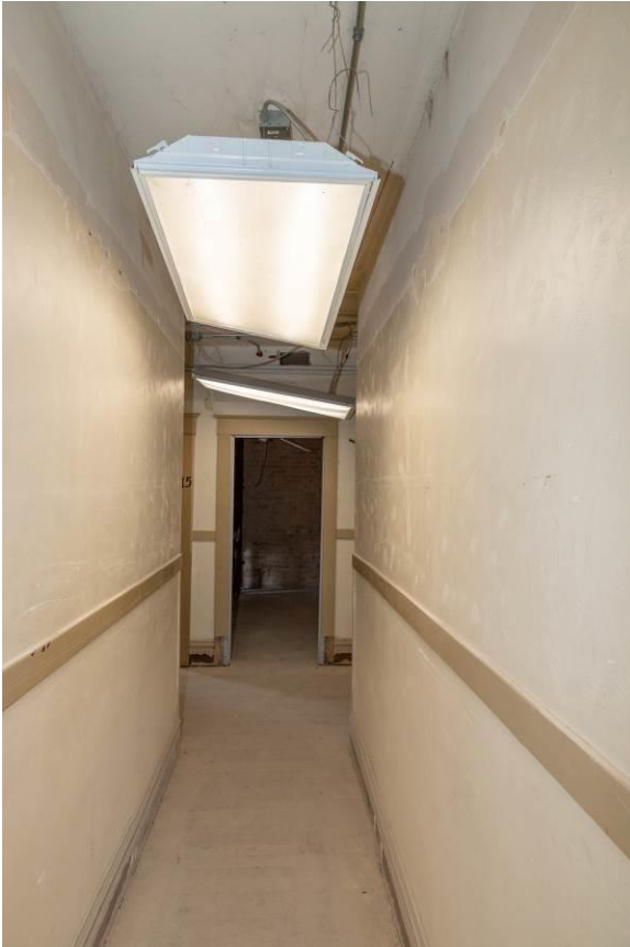
WA_Spokane County_Hotel Collins_0032. Second floor, typical branch hallway, looking west towards the main hallway.
