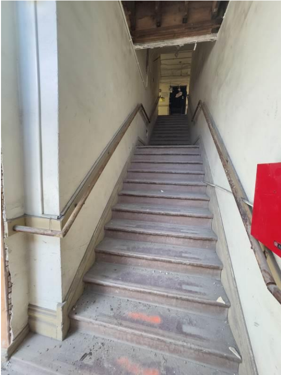
WA_Spokane County_Hotel Collins_0022. First floor, central stairway, looking up from the 204 South Wall Street entrance.
