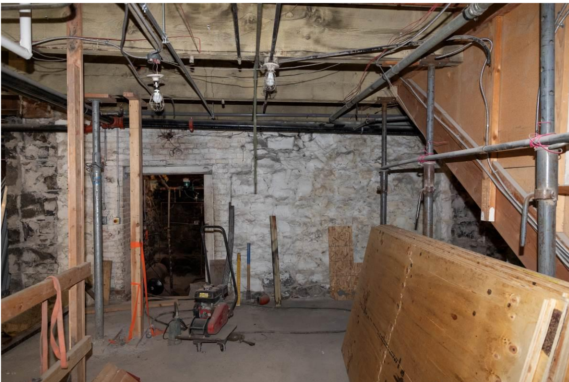
WA_Spokane County_Hotel Collins_0013. Basement, looking west towards the boiler room doorway.
