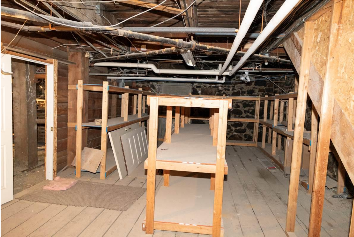
WA_Spokane County_Hotel Collins_0014. Basement, below the 212 South Wall Street commercial space, looking east.
