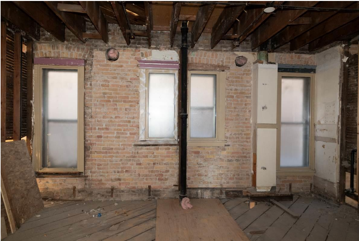
WA_Spokane County_Hotel Collins_0029. Second floor, looking west within the former shared restroom and laundry space.
