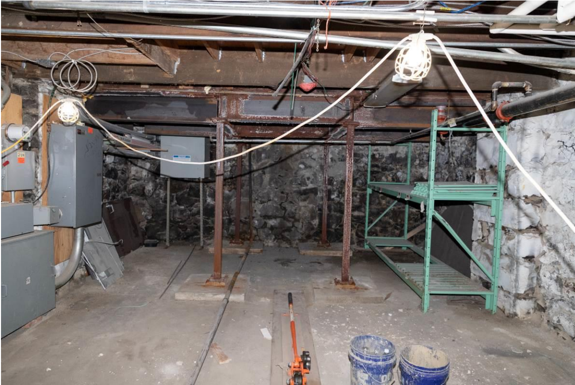
WA_Spokane County_Hotel Collins_0012. Basement, electrical space, looking northeast, with the areaway space in the background, right of the electrical panels.
