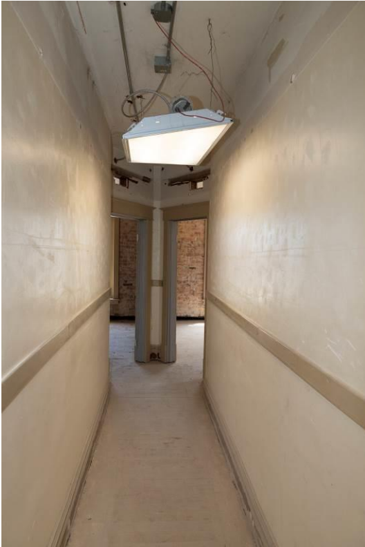
WA_Spokane County_Hotel Collins_0030. Second floor, typical branch hallway extending east of the main hallway.
