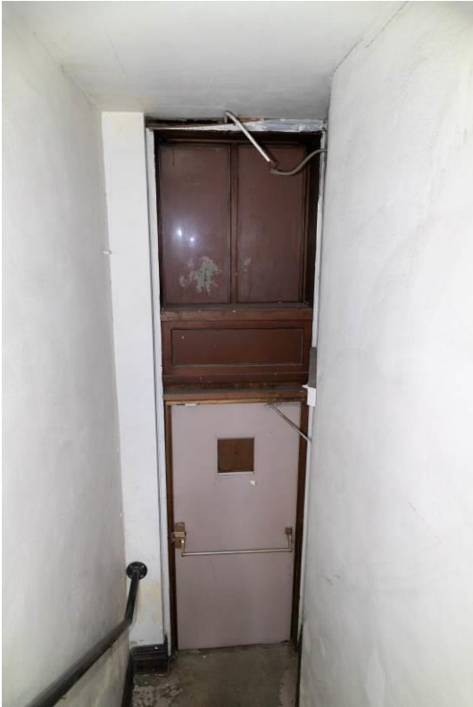
WA_Spokane County_Hotel Collins_0038. Second floor, northwest stairwell, down up from the intermediate landing at the 705-1/2 West Second Avenue entrance.
