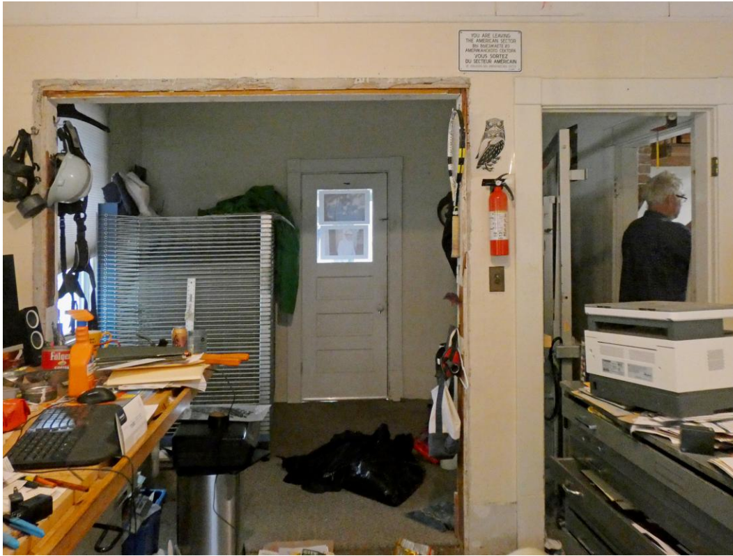
Photo 8 of 11. Former office reception area (foreground) and office space (background). This area was once remodeled into a kitchen with a portion of the wall separating the two spaces cut out.
