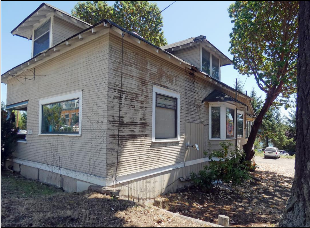
Photo 4 of 11. West face of the house. The repair in the center was where the fireplace was removed.
