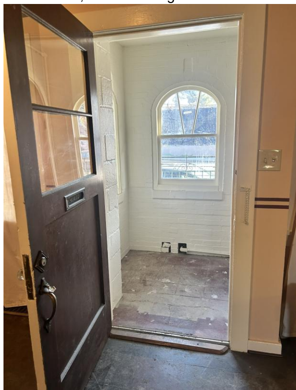
11 of 16: Detail of front door on leading into entry vestibule, camera facing east.
