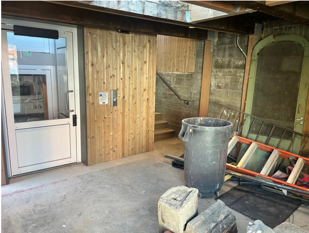
15 of 16: New addition ADA lift (left) and new addition stairwell (right), camera facing southeast.
