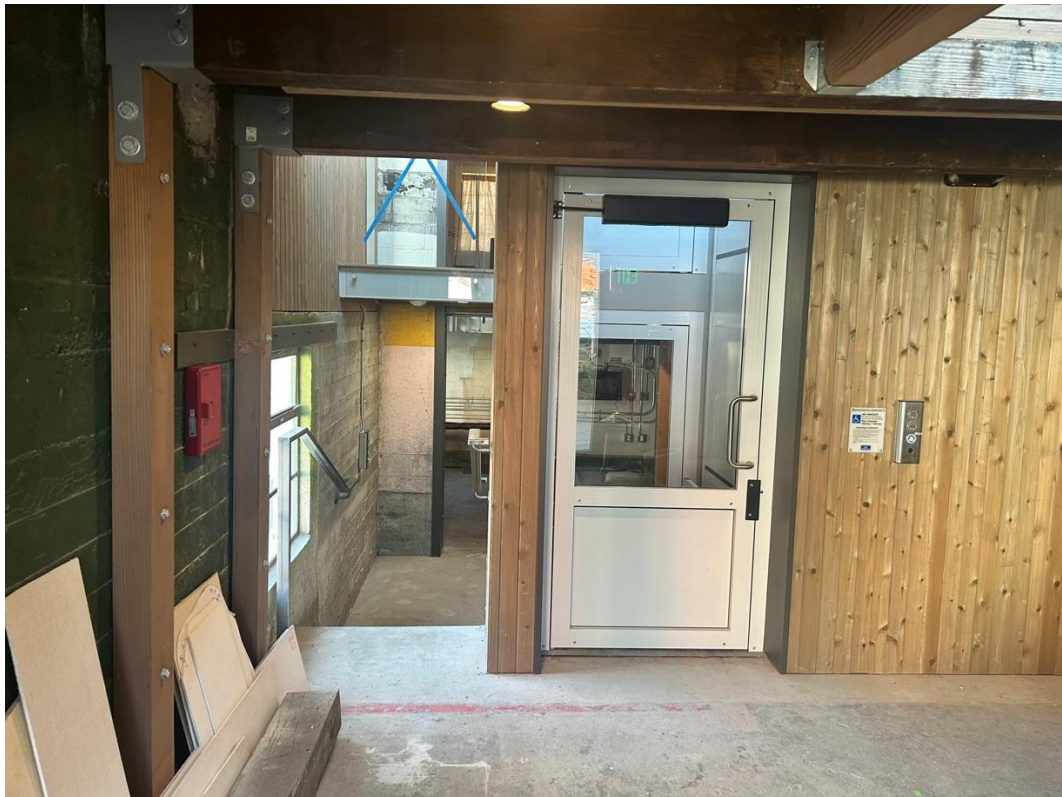
14 of 16: Hallway to basement (left) and new addition ADA lift (right), camera facing east.
