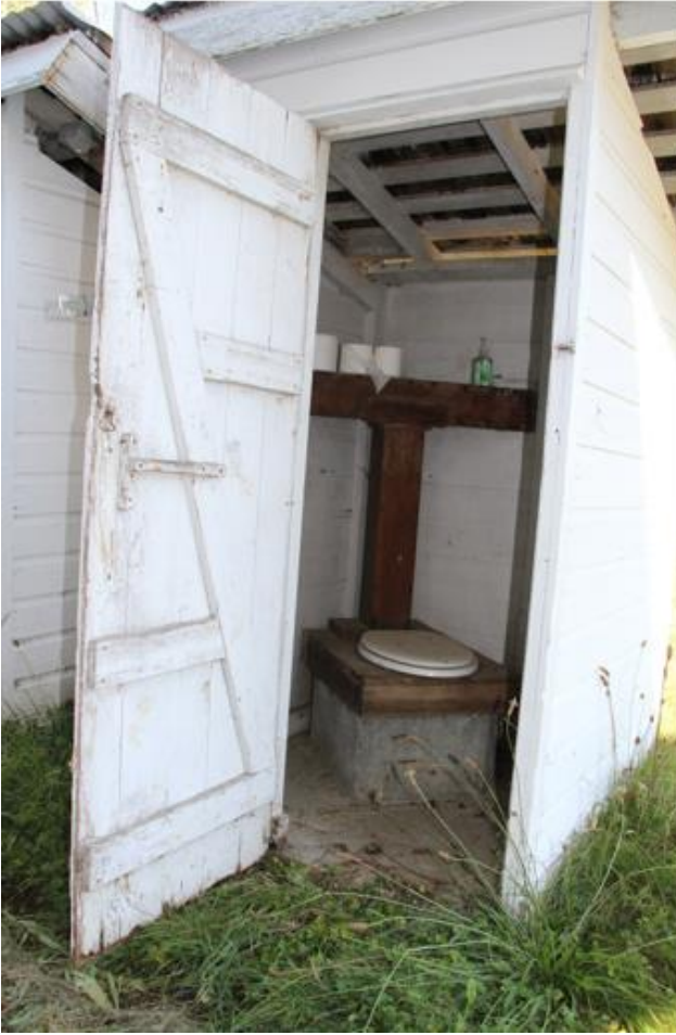
6 of 14. Front (west) elevation facing east of circa 1930s WPA-era outhouses. Photo labeled as WA_SkagitCounty_HoogdalSchool_6.
